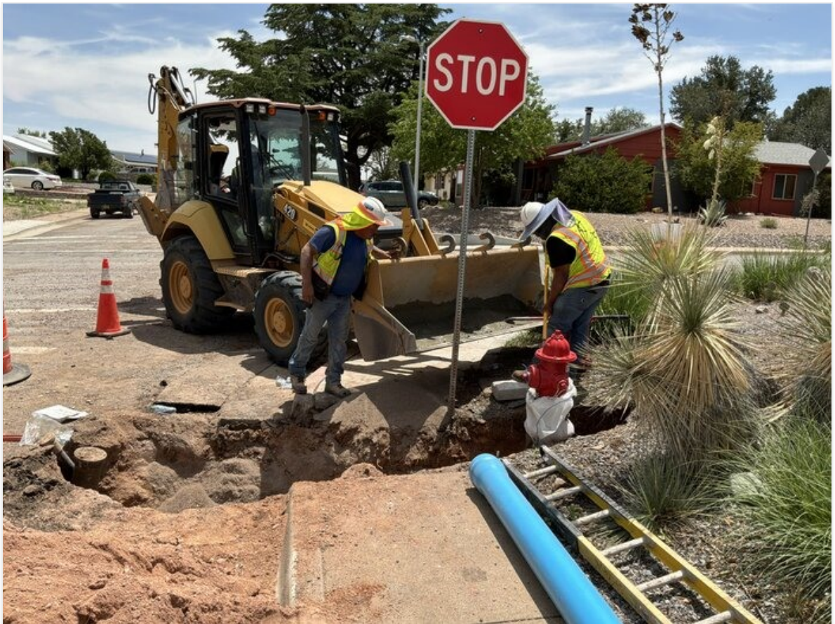
New hydrant on Cuprite Ave.
