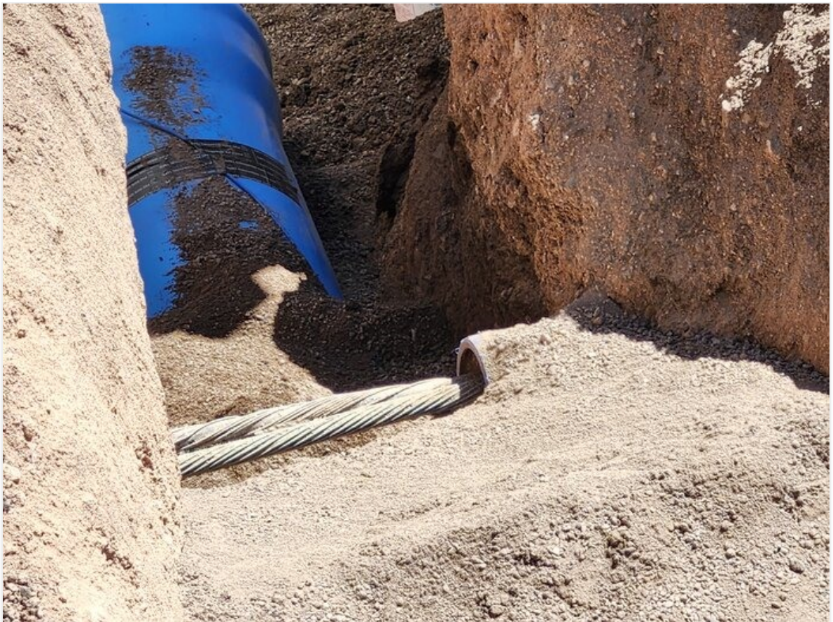
Unmarked existing dead power line at sta. 22+00.
