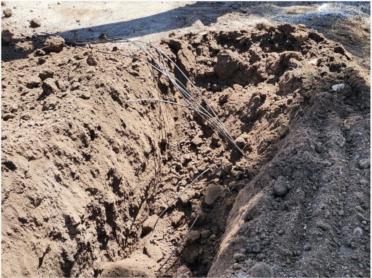
Exposed and broken communication lines on Copper Dr. sta. 57+05. Lines are old and dead.
