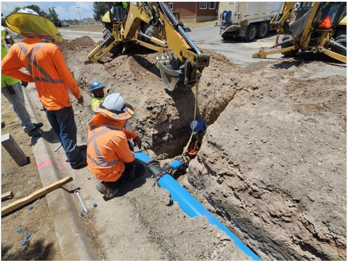
12x6 tee for fire hydrant #2 on Copper Dr.
