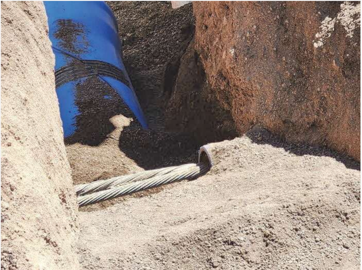
Unmarked existing dead power line at sta. 22+00.
