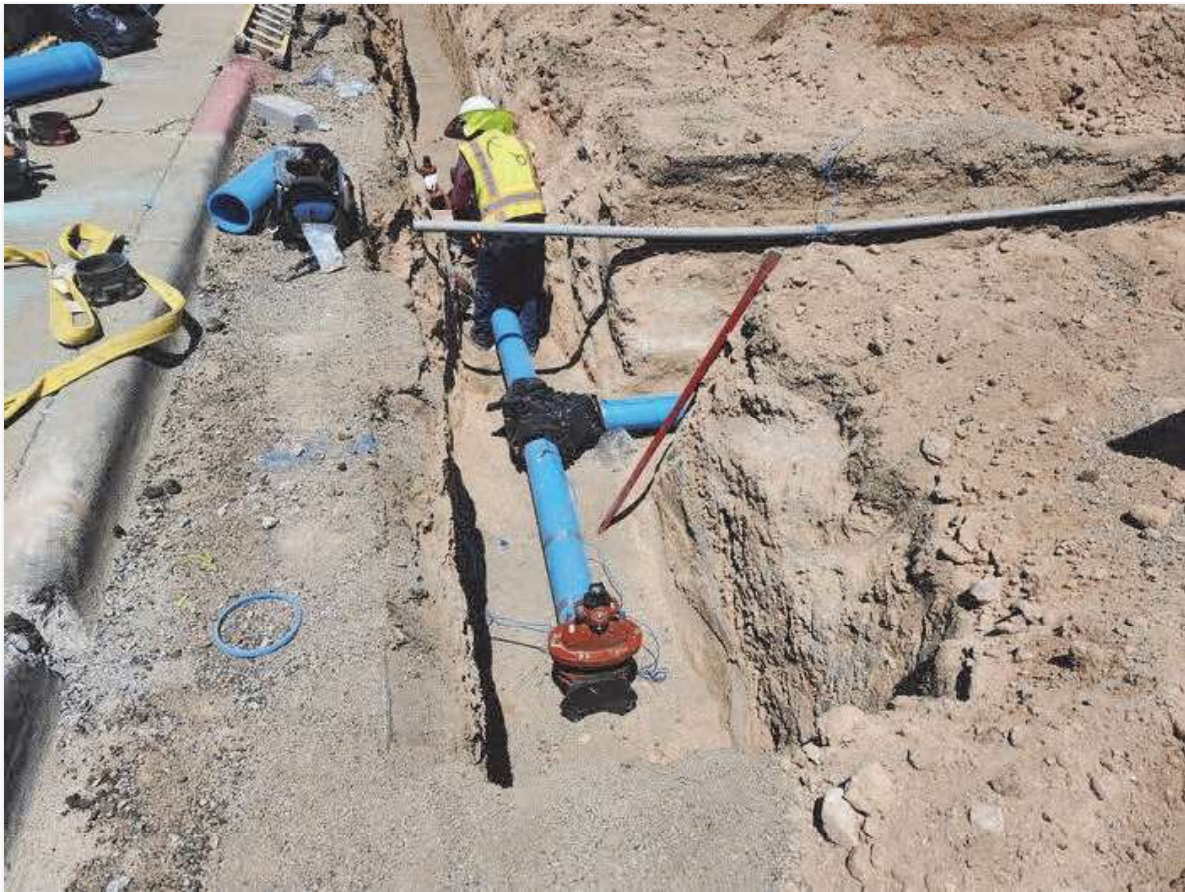
Tee with GV wrapped in anticorrosion plastic on Covellite Dr.
