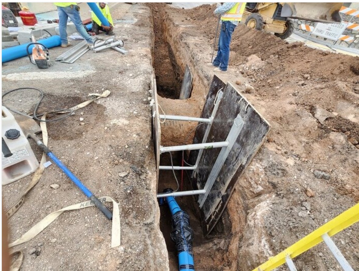
45 DI bends under 48" storm drain on Copper and Chalcopyrite. Shoring needed.
