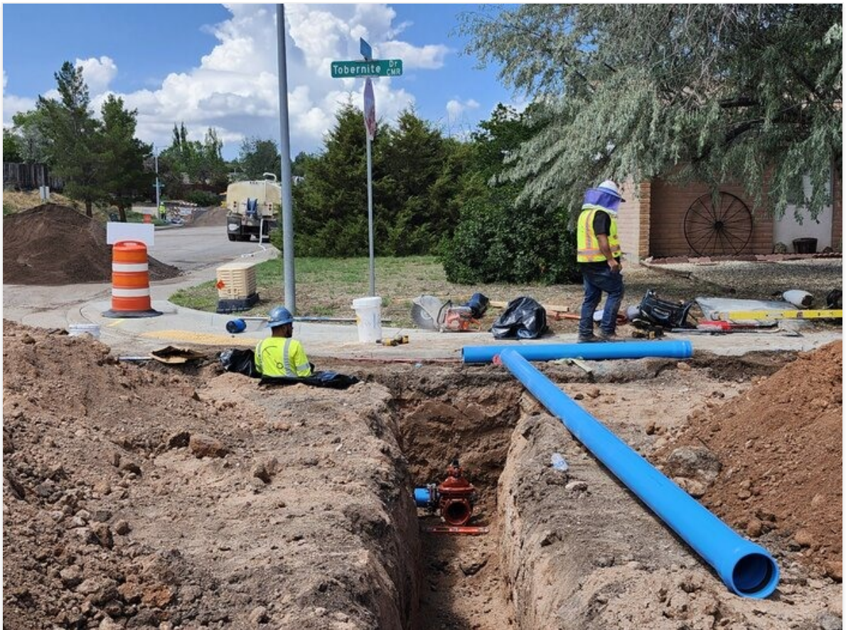
6" C-900 fire line with valve at Tobernite.
