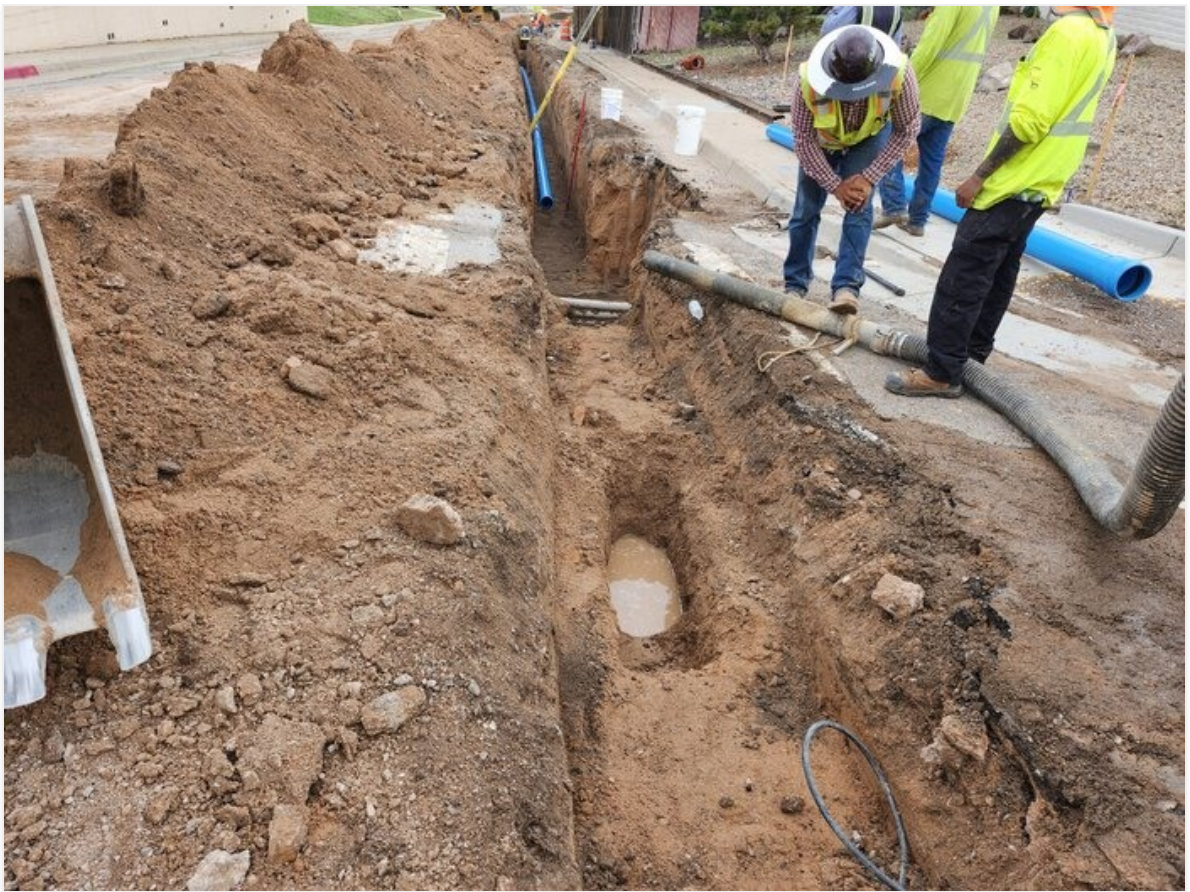
discovered existing water line leak at Cuprite and Chalcopyrite Ave.
