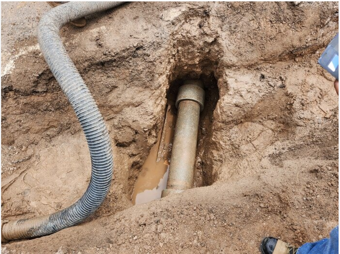
Leaking AC water line joint.
