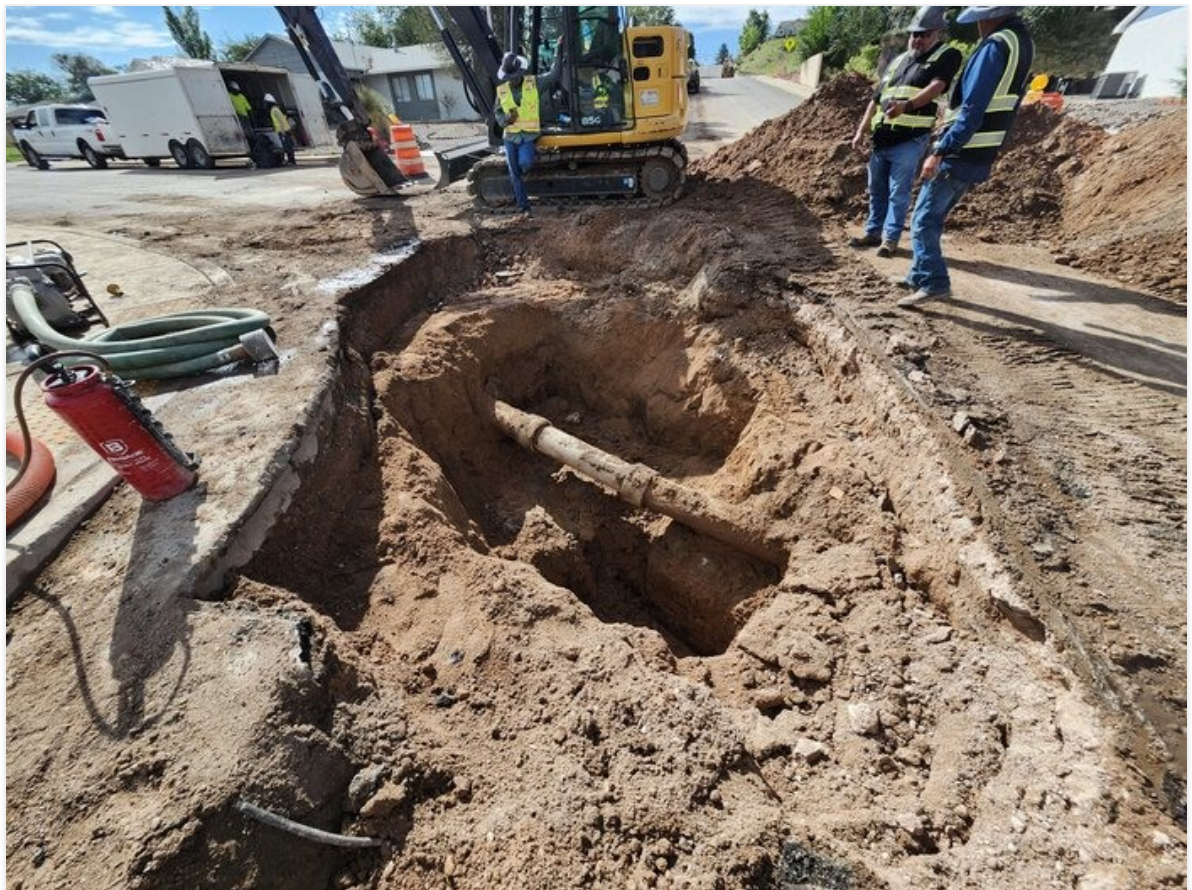
Exposed leaking 8" AC water line.
