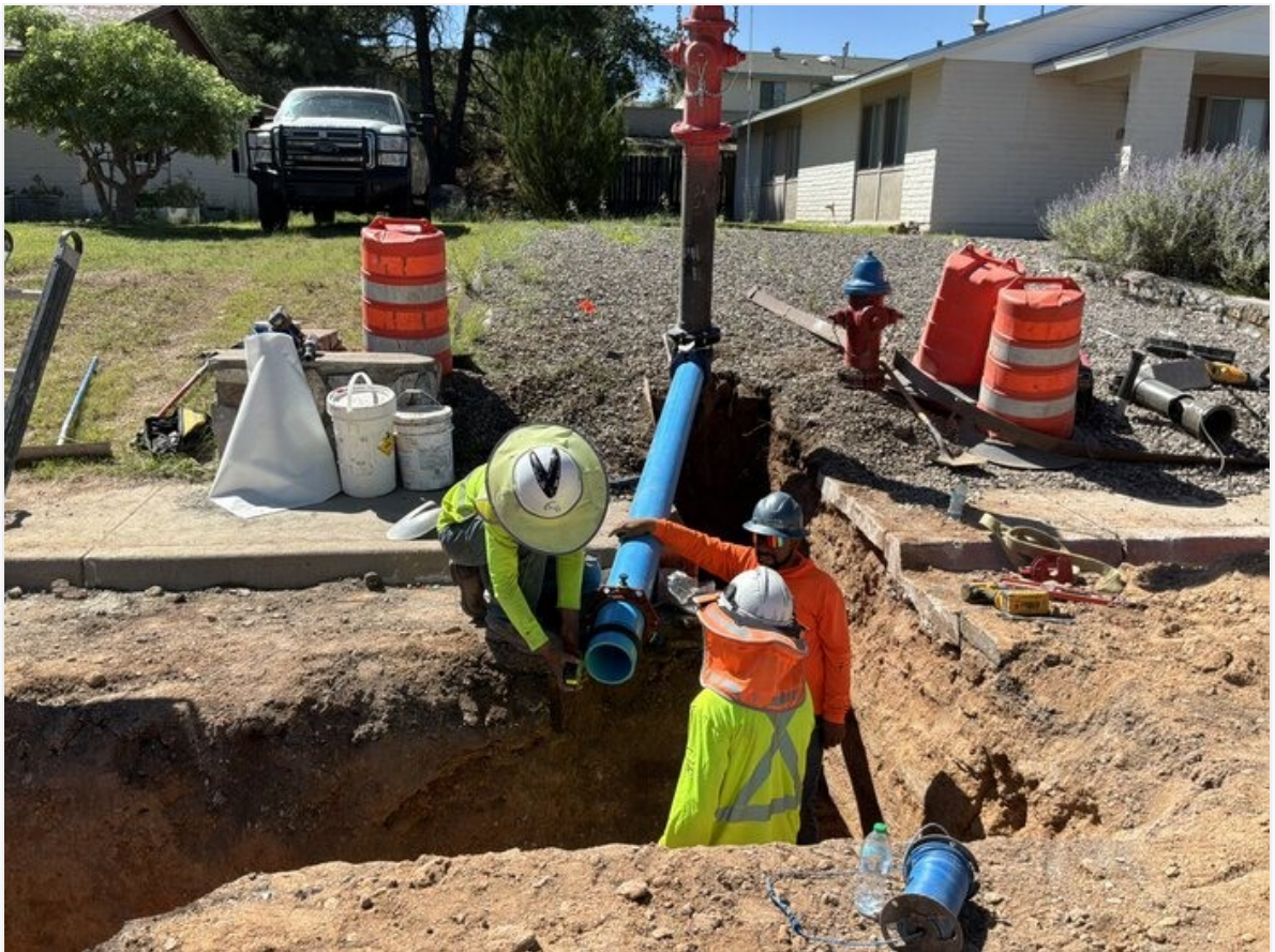
Hydrant placement on Bornite St.
