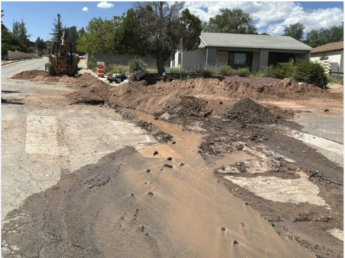
Damaged water line on Bornite St. sta. 26+80
