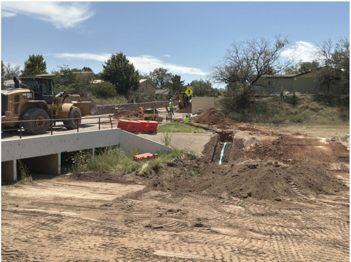
Caution tape at removed concrete sloped blanket.
