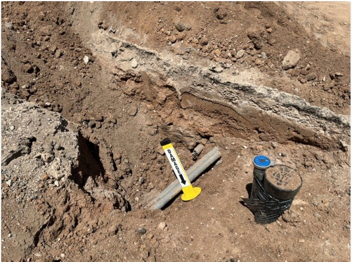
Damaged unmarked communications line on Bornite St. sta. 23+65
