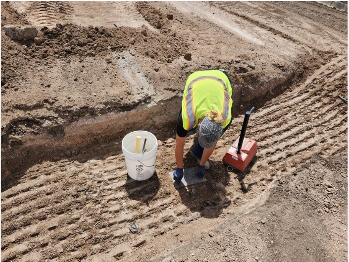
Testing lab taking densities over backfill on intersection of Cooper Dr. and Cuprite St.
