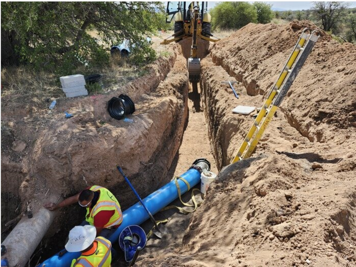
12" C-900 under existing AC water line with slight alignment shift away from existing line.
