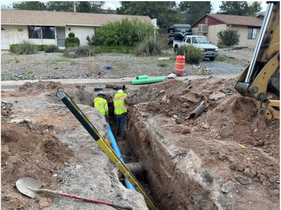
Fire line on Cuprite St. at approx. sta. 29+17
