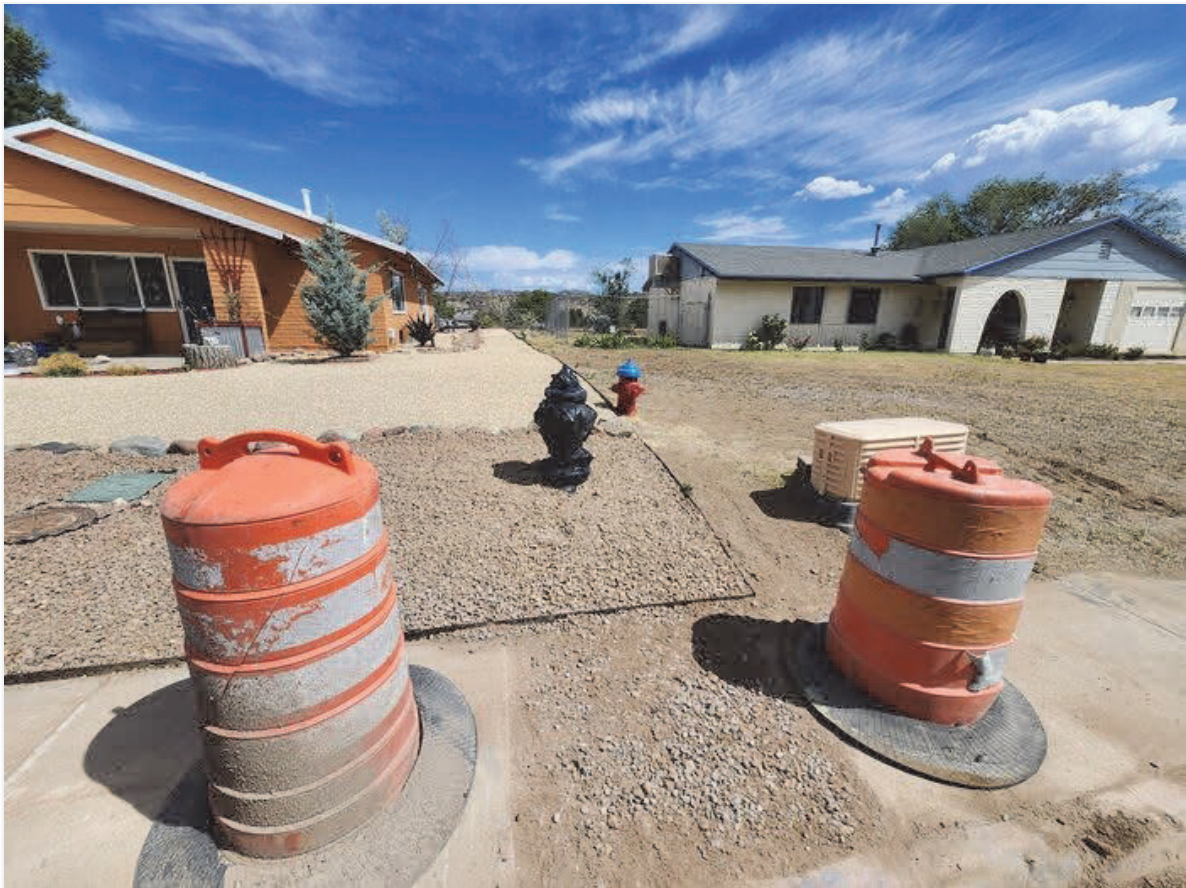
New hydrant placed on Chalcocite St. covered with black bag.
