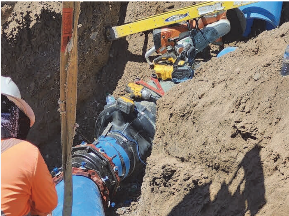
Rubber boot with clamps at east end of 24" steel casing on Copper Dr. arroyo.
