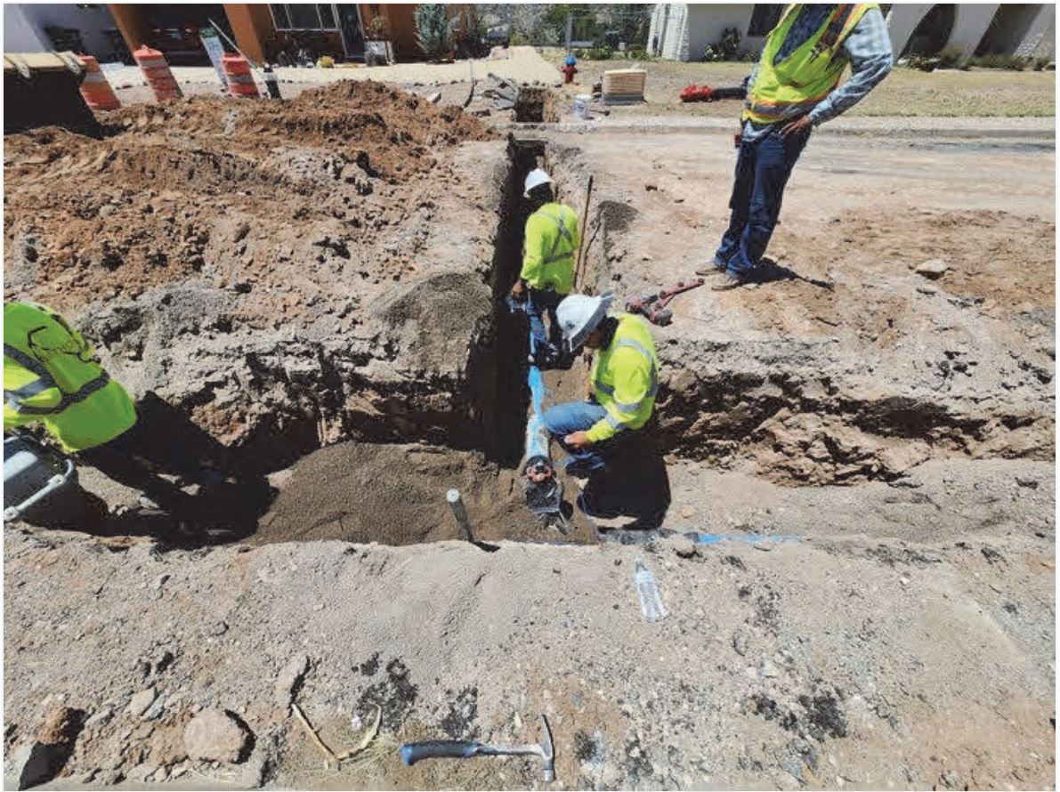
6" C-900 and fire line on Chalcocite St.
